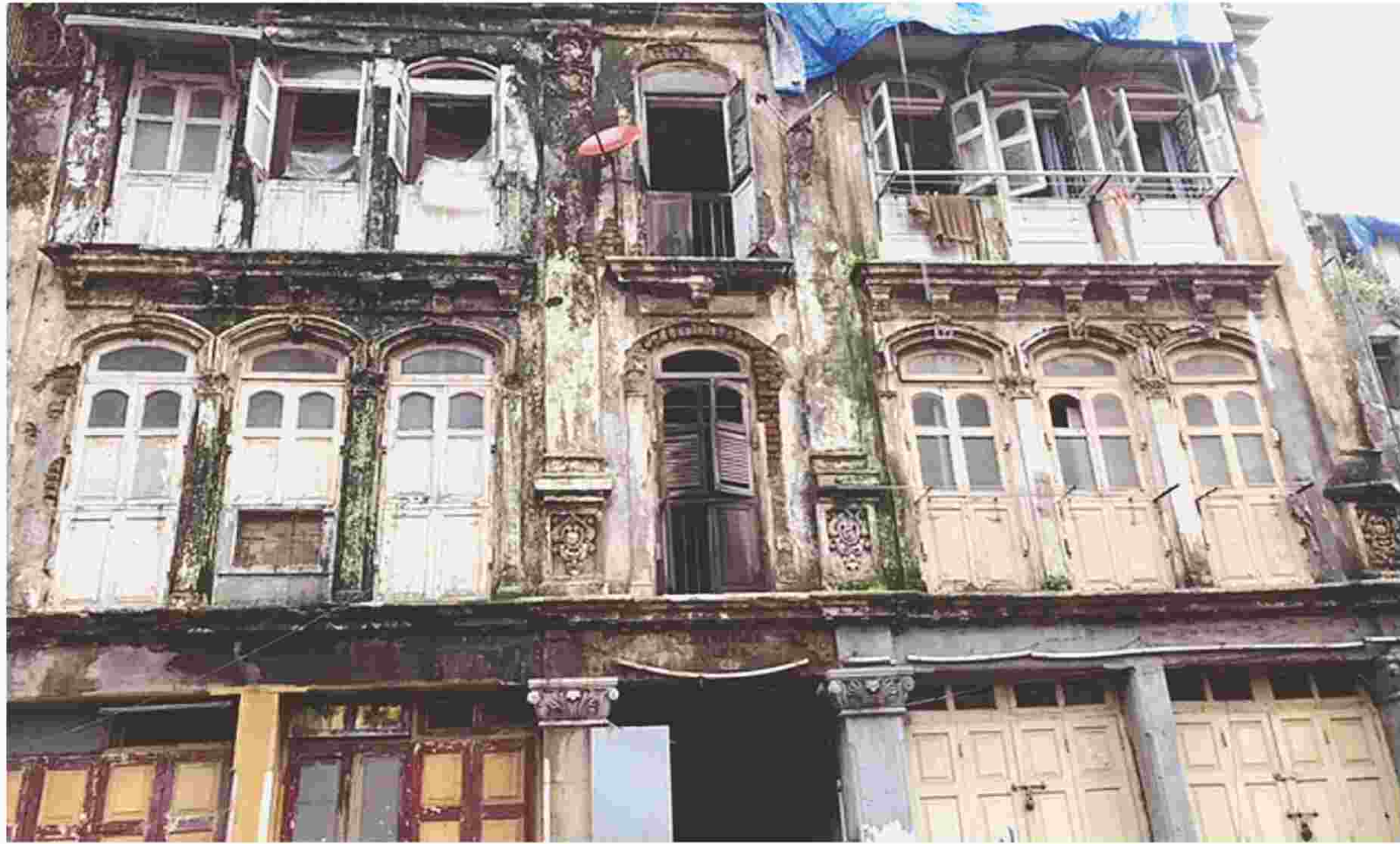
DILAPIDATED colonial-era buildings in Mumbai's Bhendi Bazaar.—ANN
