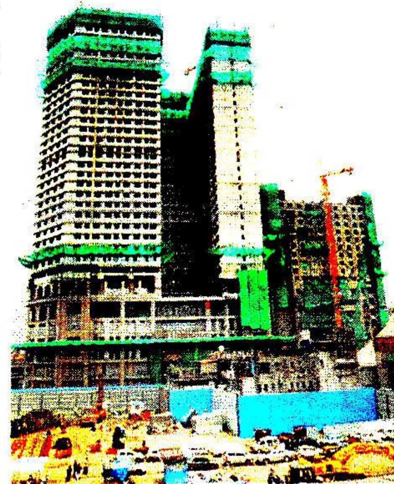
Work on sub-clusters I and III of the project is expected to be completed by mid-2019
